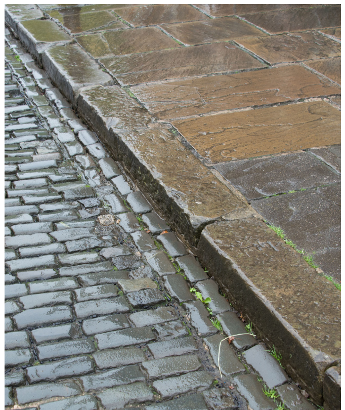
Walk around or inspect your premises to identify slip and trip hazards.
